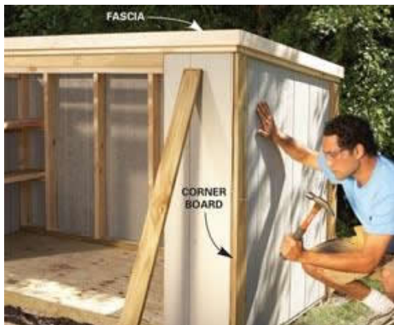
PHOTO 7: NAIL ON THE TRIM
